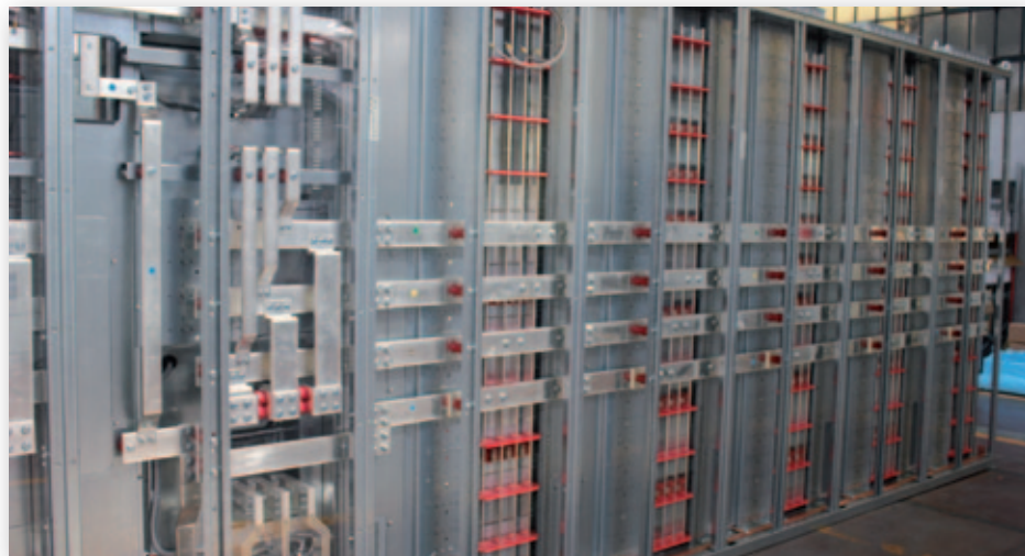
Retro sbarre omnibus e calate verticali Back omnibus busbars and vertical drop
